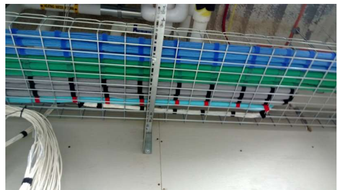
Figure 17: Cable and Wiring (4)
