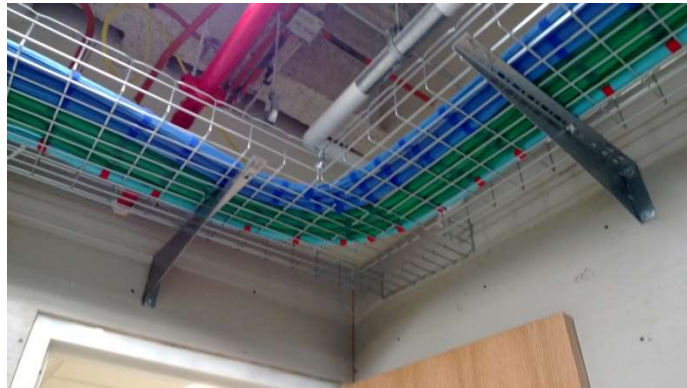
Figure 18: Cable and Wiring (3)
