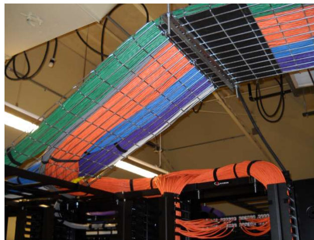
Figure 19: Cable and Wiring (1)
