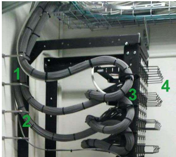
Figure 16: Cable and Wiring (2)
